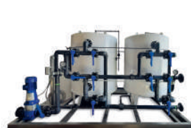
WATER TREATMENT PLANTS. FILTRATION
